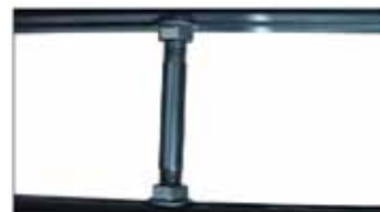
Fig 2. Connection of upper to lower profile by means of stud bolts which are fastened with a self locking nut.
